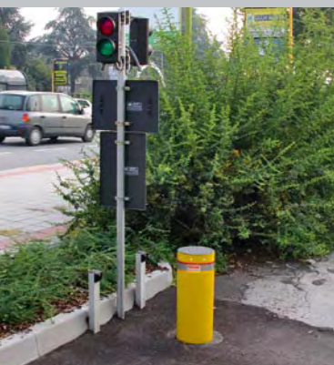
Strabuc 918 with Polo 44 photoelectric cells and indicator traffic lights
